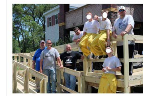
A crew from the Logansport Juvenile Corrections facility, along with their Indiana Department Of Corrections supervisor built a SAWs ramp for a 58-year-old man with COPD, Parkinson's and CHF. Seeing the impact building a SAWs for those in need can have a transformational impact on the lives of young offenders.
